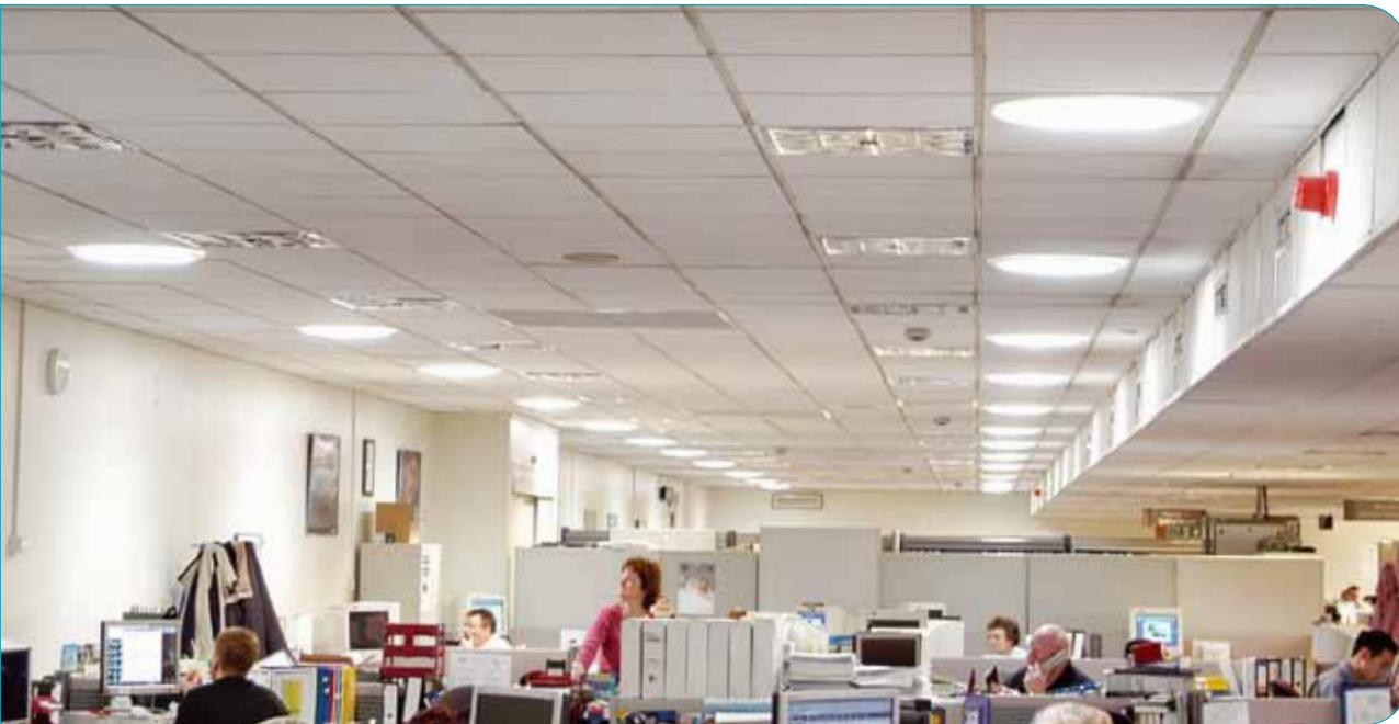
Above: Internal view of Windcatchers and Sunpipes installed at the Daimler Chrysler offices in Milton Keynes
