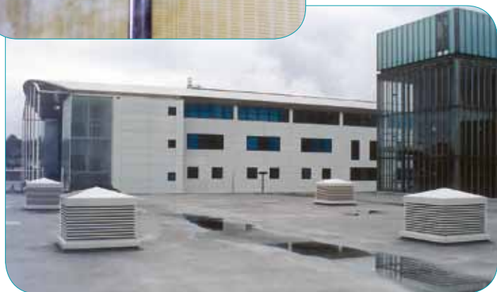
Below: Windcatcher units installed on flat roof of old central mainframe computer building
